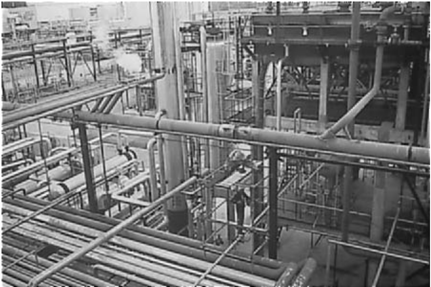
FIGURE C7.3 Typical process plant piping.
